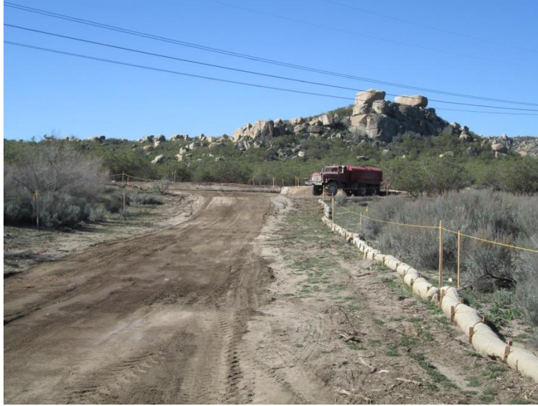
Photo 3: In accordance with MM-HYD-1 and the East County Substation Stormwater Pollution Prevention Plan (SWPPP), straw-wattles have been placed along the work limits to minimize the potential for erosion to be discharged offsite.
