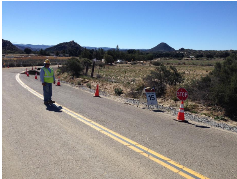
Photo 2: In accordance with MM-TRA-1, flaggers and signage are being utilized along Jewel Valley Road to ensure the safe passage of motorists during construction activities.
