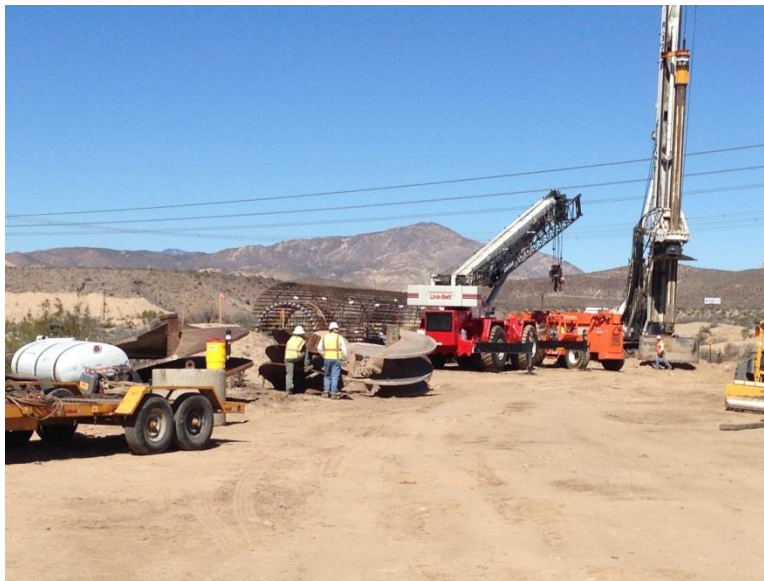
Photo 4: Construction crews were observed completing drilling activities within the approved work limits at steel-pole 90 in accordance with MM-BIO-1a.
